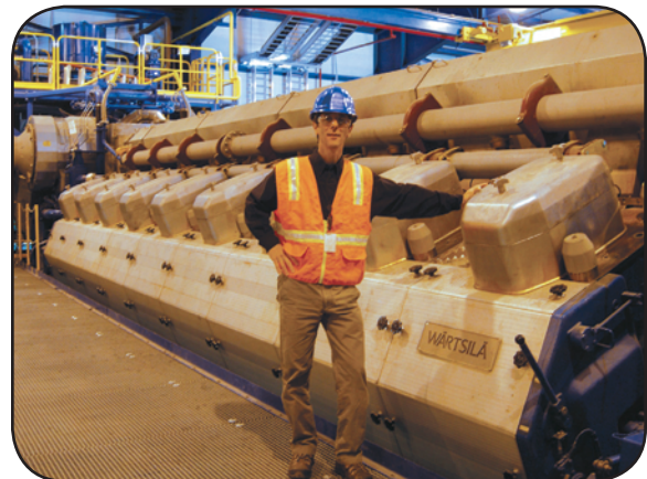
RESCO Project Manager Jim Zoellick stands next to a 10 MW Natural Gas generator, one of sixteen that were recently installed by PG&E to replace the aging power plant at King Salmon south of Eureka. The generators will be a good match to intermittent renewable energy like wind and wave power.
